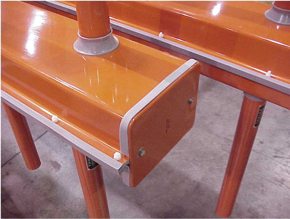
Figure 1.0. Example of Improper Installation of Gasket
